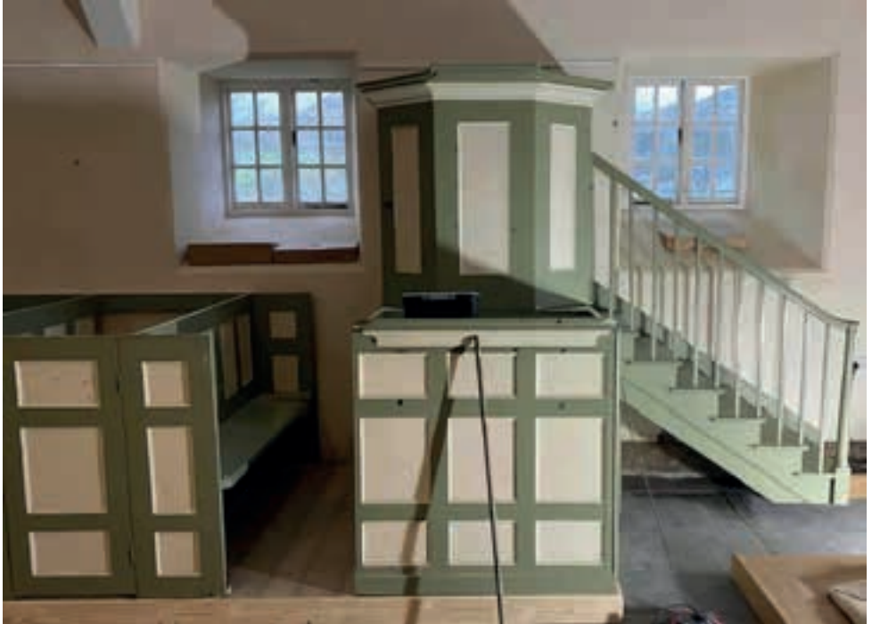
The pulpit and reading desk back in position on the north wall, awaiting full restoration and a new pew door.
